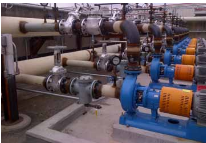
Ethanol railcar unloading pumps in Albany NY
