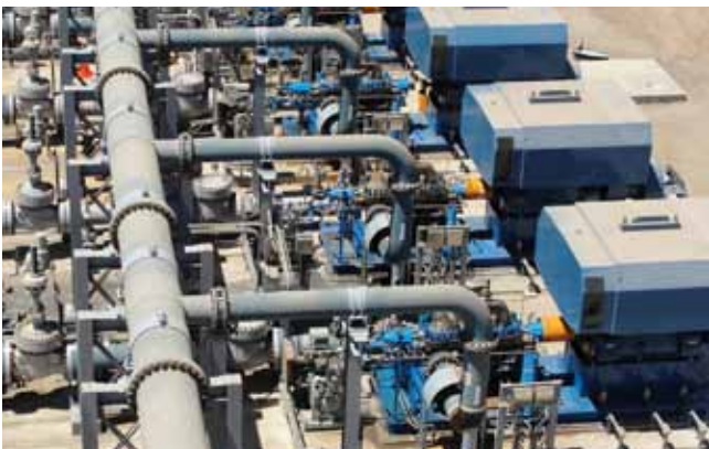
Twenty Model 3600 API pumps propel seawater 90 miles from the Pacific Ocean to a copper mine
