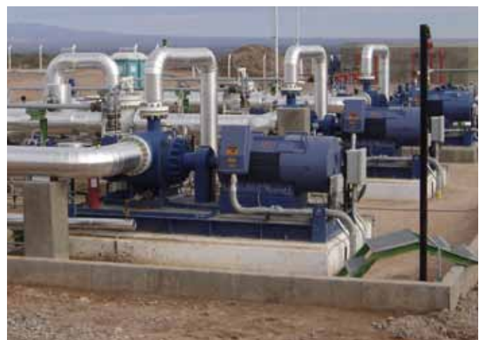
Heavy crude oil transfer pumps with viscosities ranging from 50 to 900 cSt. When "frozen," this pipeline relies on ITT Bornemann twin screw pumps
