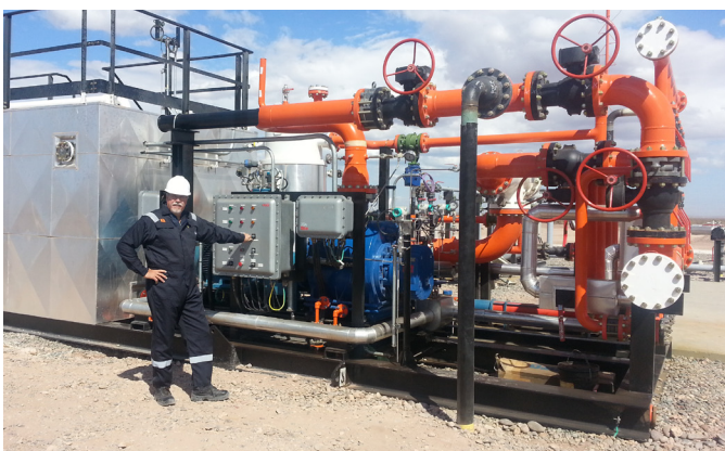
A mobile, multiphase pump system that can handle the oil, water and gas produced at wells
