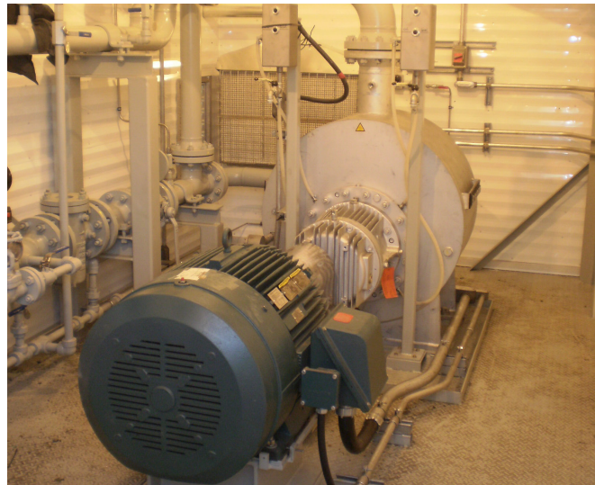
Multiphase pump installation
