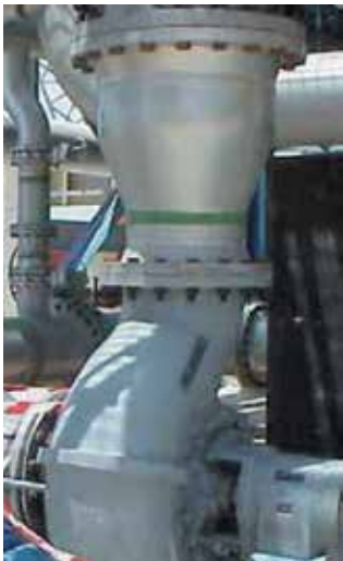
Cooling water pump for primary turbine at a power plant in the Middle East.
