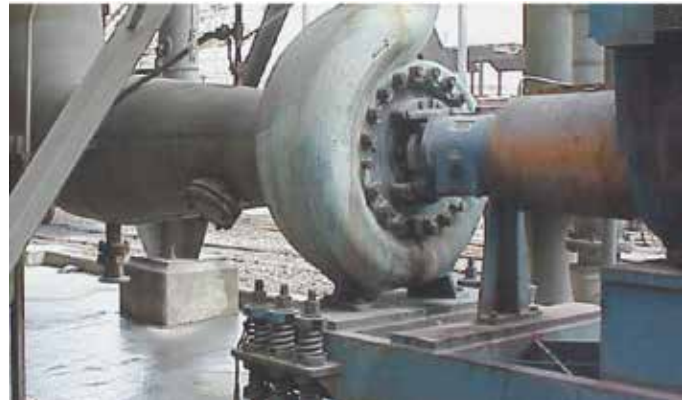
Installation for a difficult high-temperature service. Spring-mounted baseplate provided to compensate for thermal expansion.
