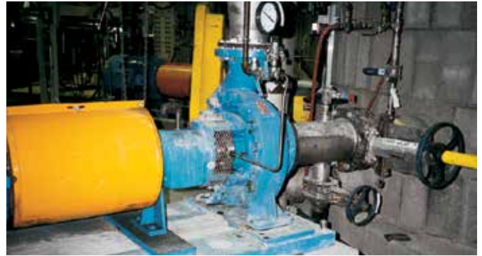
A Model 3180 installed in a North American recycle mill.
