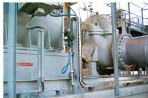
Refinery Crude Oil Service (Middle East)
