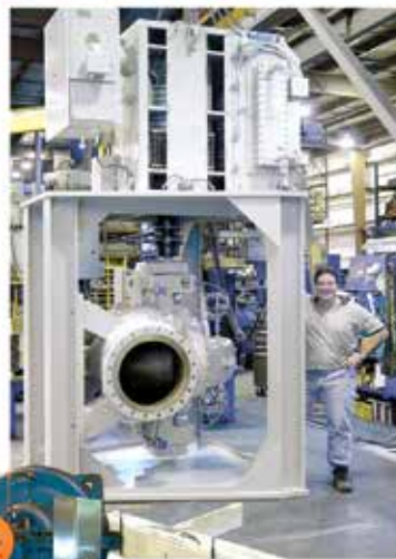
Offshore Platform Service (Gulf of Mexico)
