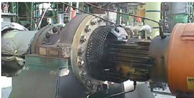
Model 3700 on high-temperature service at a U.S. Gulf Coast refinery.
