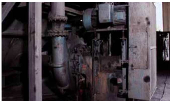
Overhead motor-mounted Model 5500 in a coal preparation plant – heavy media cyclone feed service.
