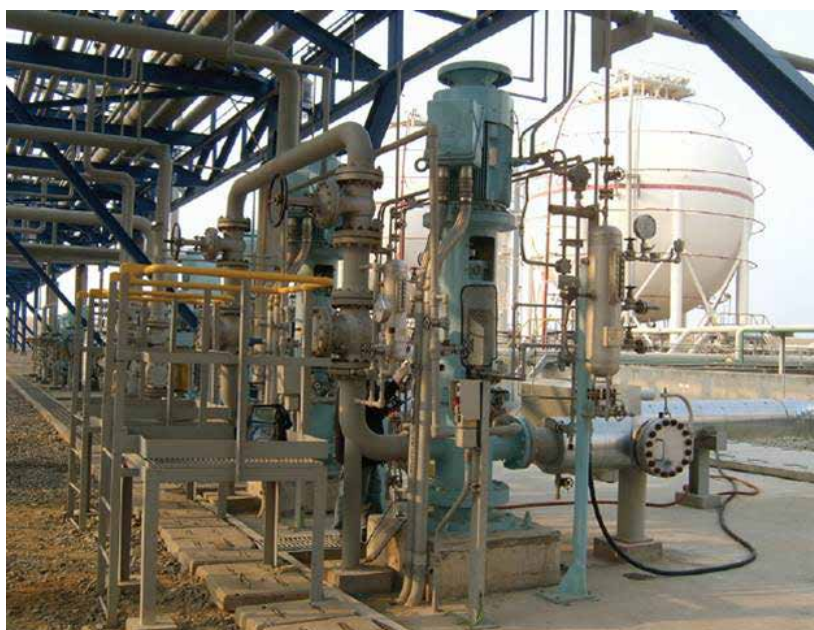
Many of these high head applications involve pumping low specific gravity hydrocarbons in a VS6 suction can arrangement.
