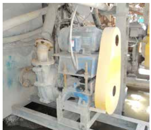
Mill discharge in silver plant
