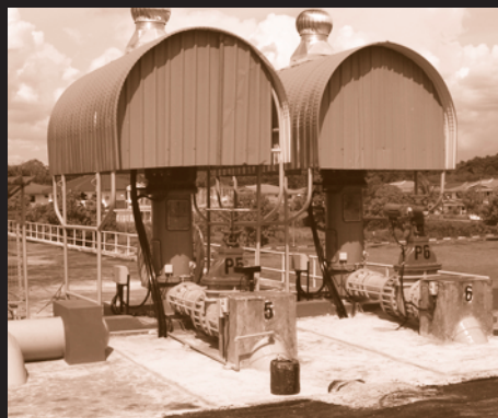
Salim Water treatment plant in Malaysia. Tag No. 5 and 6 (Goulds VIT) - zone 60.
