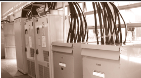
Two PumpSmart PS200 controllers.
