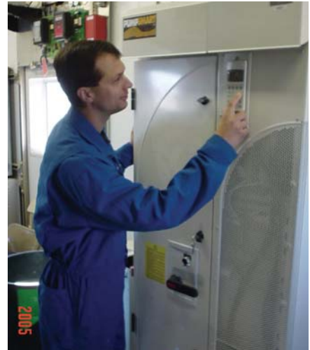
Enterprise Engineer, Kevin Dostal, checks the power draw from the PS200 key pad.
