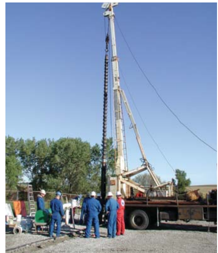
Goulds Model VIS 10JMC 28 Stage pump is lifted into place for installation.
