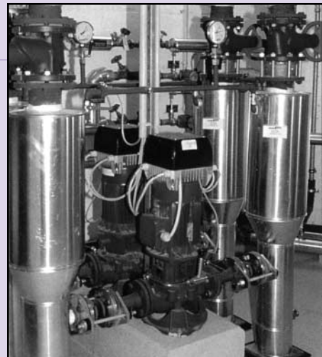
Figure 2. Theiss Power Station utilizes twenty three Hydrovar™ equipped pumps to control operating costs.
