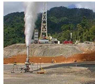
Lihir Geothermal Power Plant
