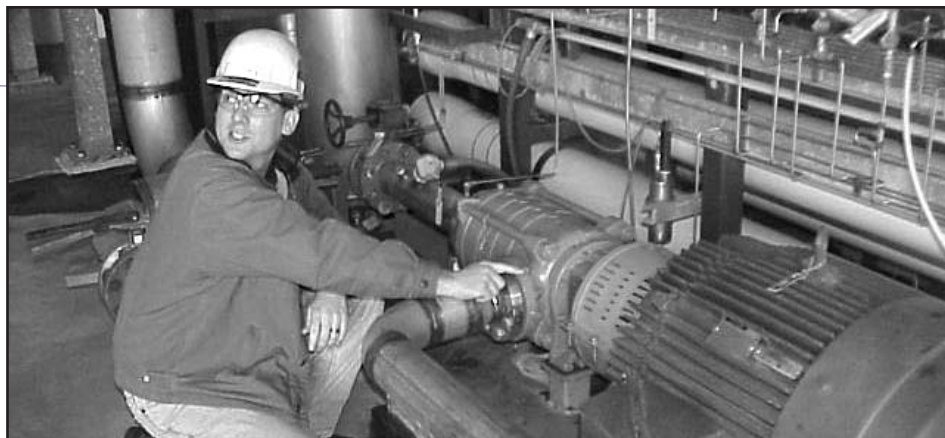
Chris Jones of Brownlee Morrow Engineering points to Goulds 3355 multistage RO pump.
