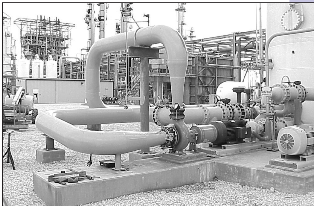
Air Products 3196 Turbine Loop is saving $24,000 annually in energy costs.
