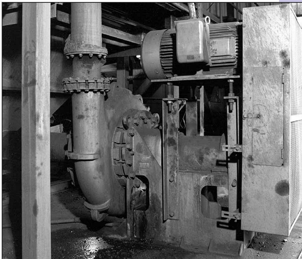
Goulds Model 5500 pump on Raw Coal Feed Service (Heavy Media Cyclone Feed).
