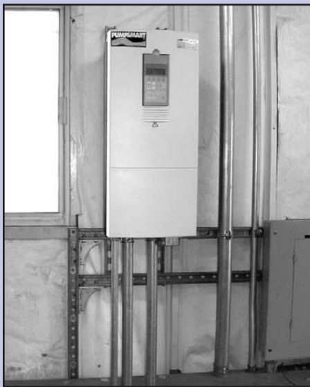
PumpSmart PS200 controls process pumps at Motiva fuel distribution terminals.
