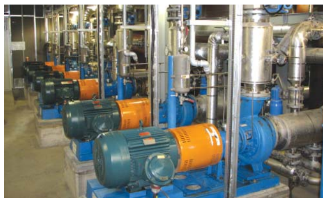
3196 in Ethanol Evaporator Service
