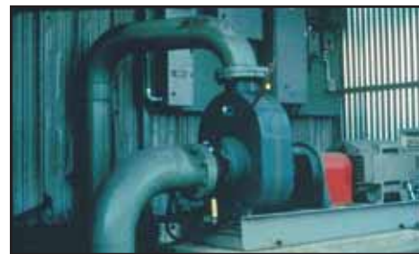
Typical Self Priming Centrifugal on Industrial Sump Service
