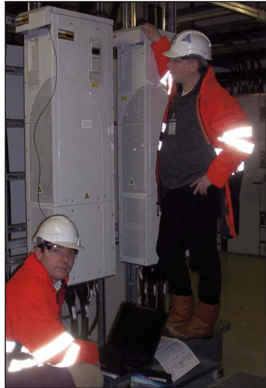
ESI team installing ITT PumpSmart system.
