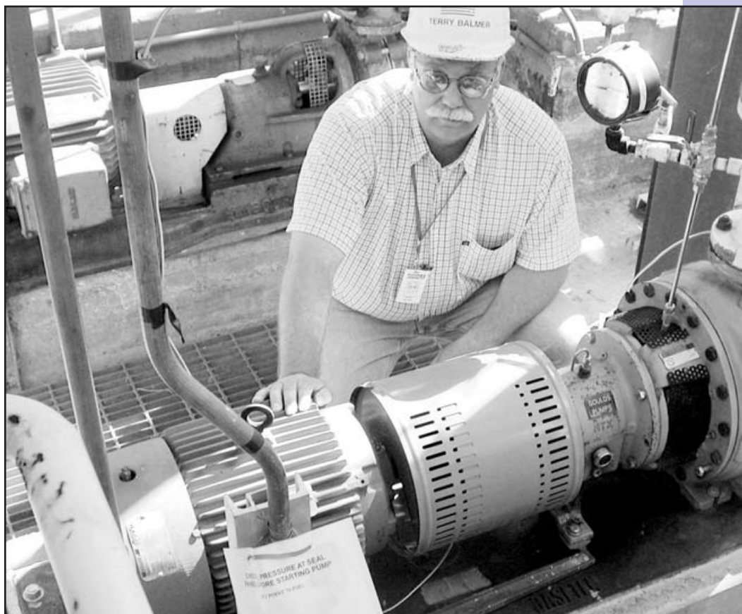
Terry Balmer of Rohm and Haas inspects one of over one hundred process pumps involved in the life cycle cost reduction program.
