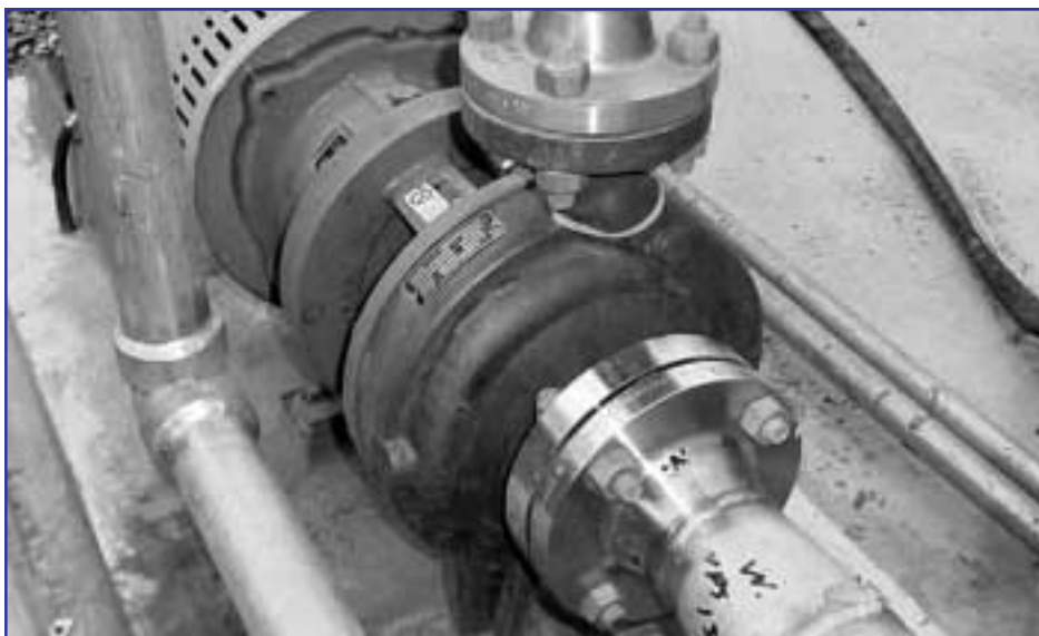
Stainless steel pump casing showing evidence of rusting due to surface contamination.
