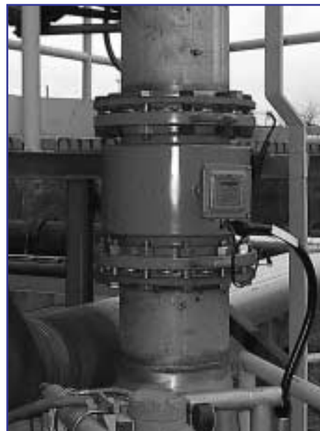
Figure 2. Flow meter replaces inefficient control valve.
