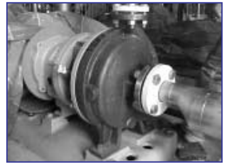
Stainless steel pump casing showing evidence of rusting due to surface contamination.
