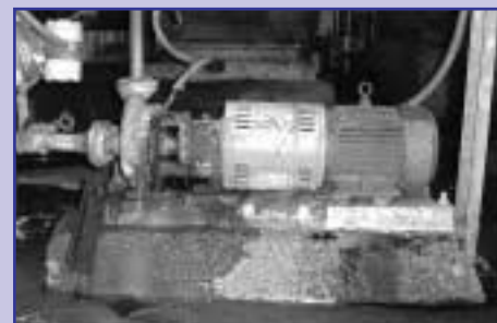
Figure 1. Standard baseplate foundation corrodes and erodes.
