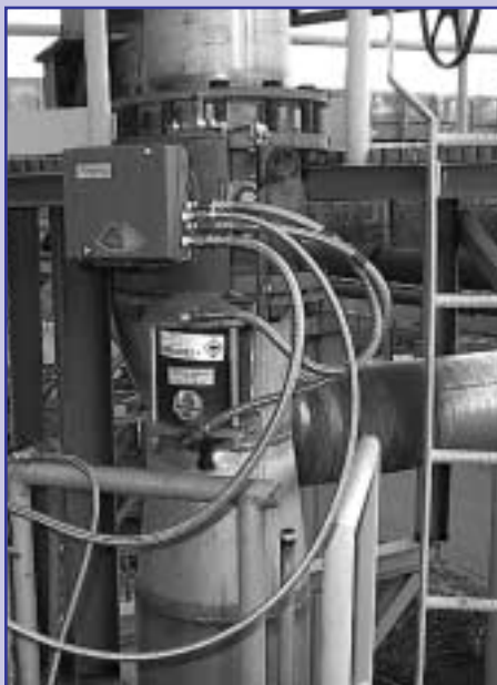
Figure 1. Inefficient valve throttling controlled flow from 200 HP fixed-speed pump.
