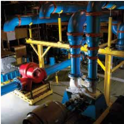
A 6000 HP / 4600 kW testing facility.
