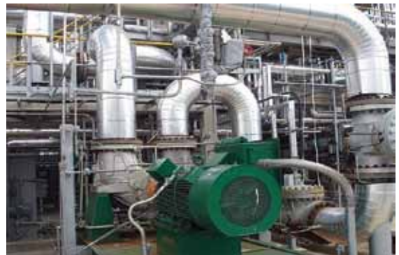
Model 3620 (BB2) boiler feedwater service located in a refinery in Asia.
