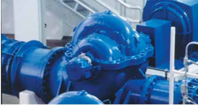
Model 3498 pumping drinking water through a distribution network in the Western United States.
