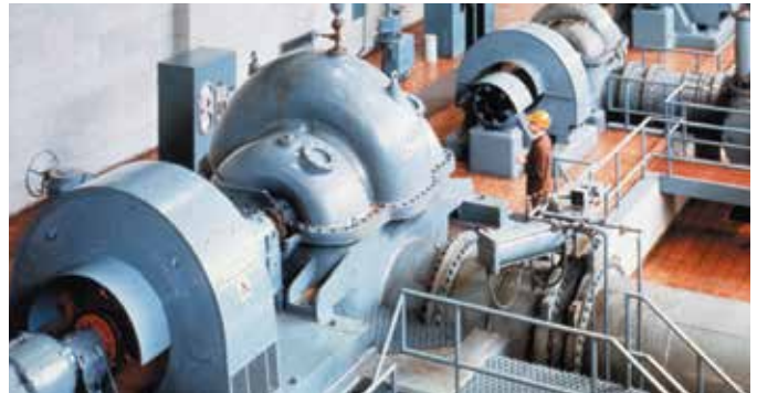
Model 3420 splitcase pump in service at an electric utility plant in the Bahamas.
