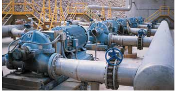
All 316 stainless steel model 3409 pumps on a solvent extraction application at a large copper mine.
