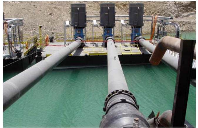
This reclaim water system at a South American copper mine employs 1300-hp pumps from ITT Goulds Pumps.
