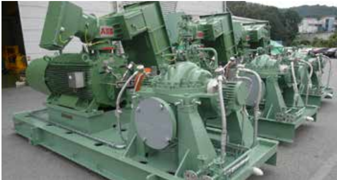
Refinery in UAE - centerline mount for higher temperatures
