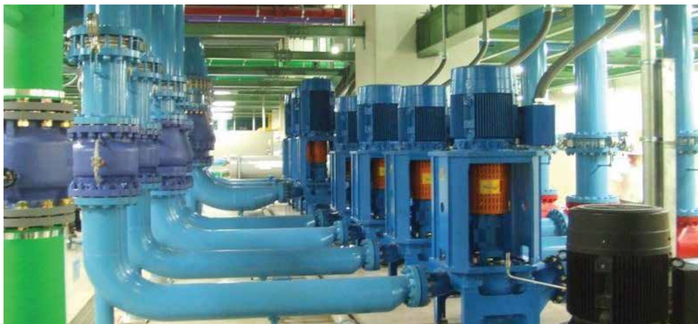
This ITT Goulds customer saved space as well as foundation and baseplates costs with seven Model 3910s. Many applications benefit from the inline piping as well.
